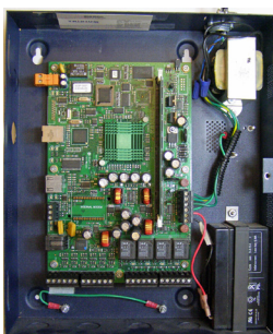
JACE-403 Before Replacement
